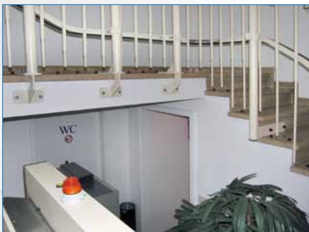
Guide rails fixed with a combination of posts fixed to the flank of the stairs, and struts in front of the risers
